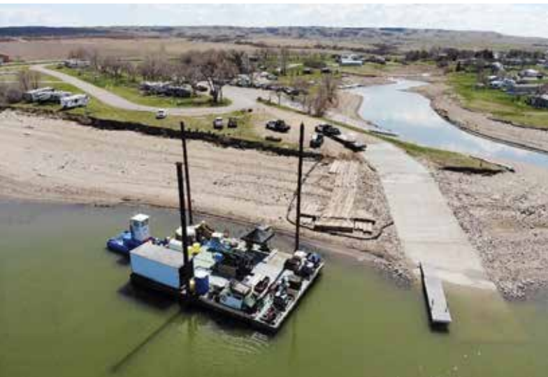
Barges were utilized for the completion of six geotechnical boreholes along the width of the lake, reaching depths of up to 315 feet below the bottom of the lake
