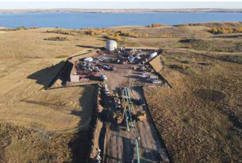
For the HDD crossing design, the entry point location was placed on the south side of the lake in a flat agricultural field
