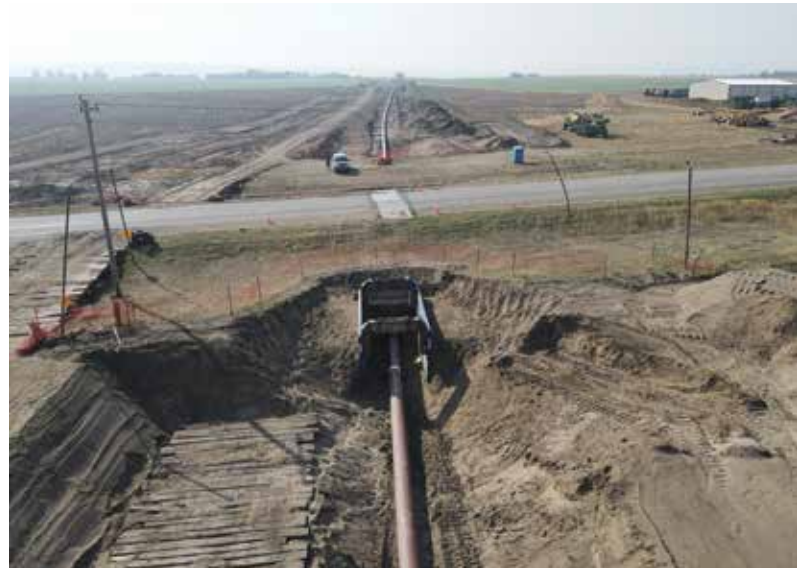
This installation, with a recorded length of 15,426 feet, marks a notable accomplishment in the HDD industry
